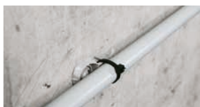
Flexible or rigid cable conduits with cable ties
