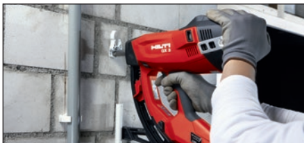
Conduits and light-duty pipes
